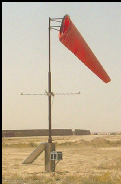
Solar Windsock Lights installed at US Army bases throughout Iraq
