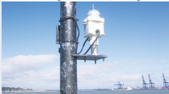
SL10 Dual Pier Lights, Harwich Harbour, United Kingdom
